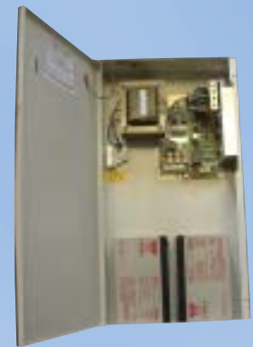
Auxiliary Power Unit provides extended back-up in the event of mains power failure.
