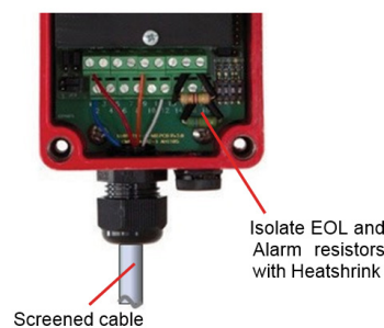
Figure 3. Control panel wiring
